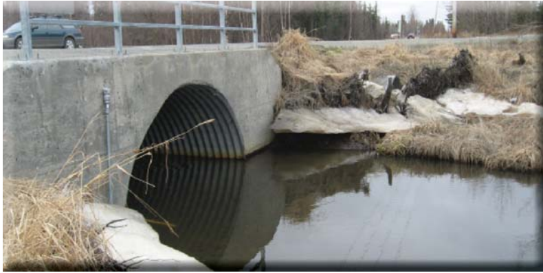
Storm drain system
