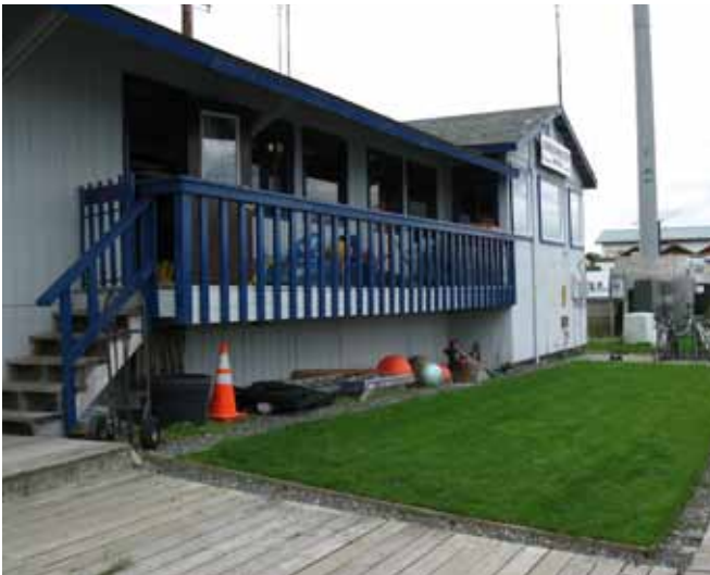
The Harbormaster's office is in poor condition, is expensive to heat, and has limited parking.
