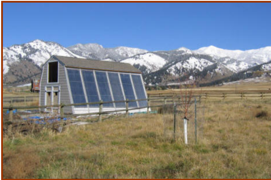
Photovoltaic collectors being used in a remote location for electricity
