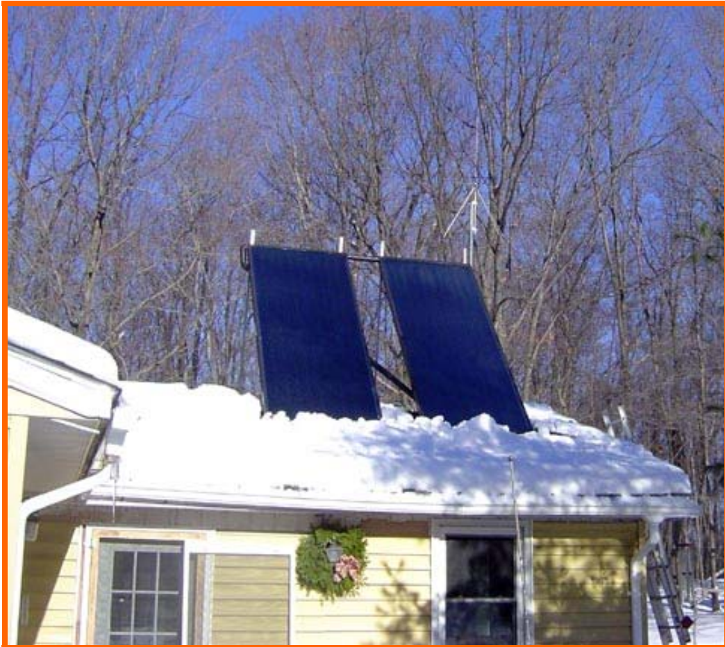
Photovoltaic collectors converting sunlight to electricity
