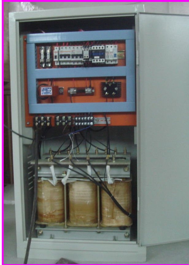
Typical Control Center
