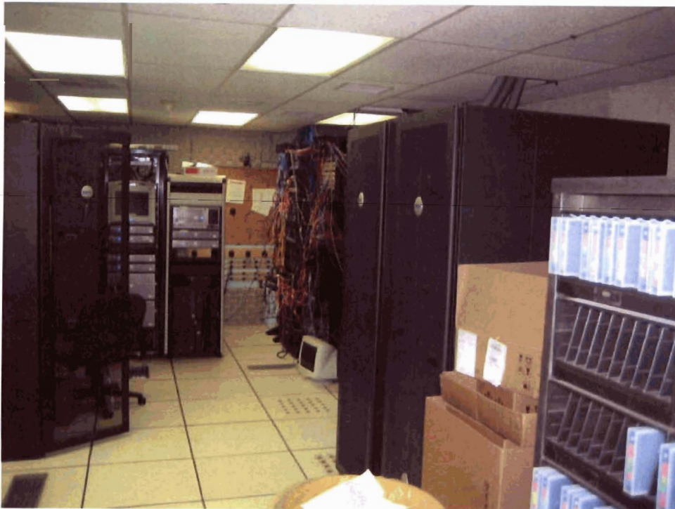
Photo 2: IT Server Room
