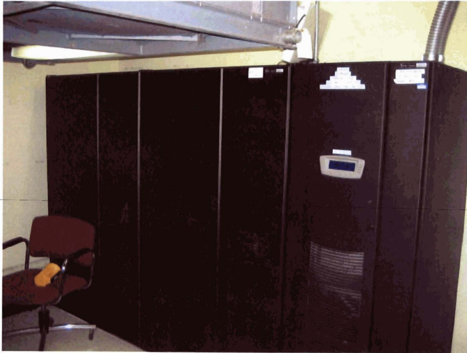
Photo 1: Existing IT Server Room AC Unit
