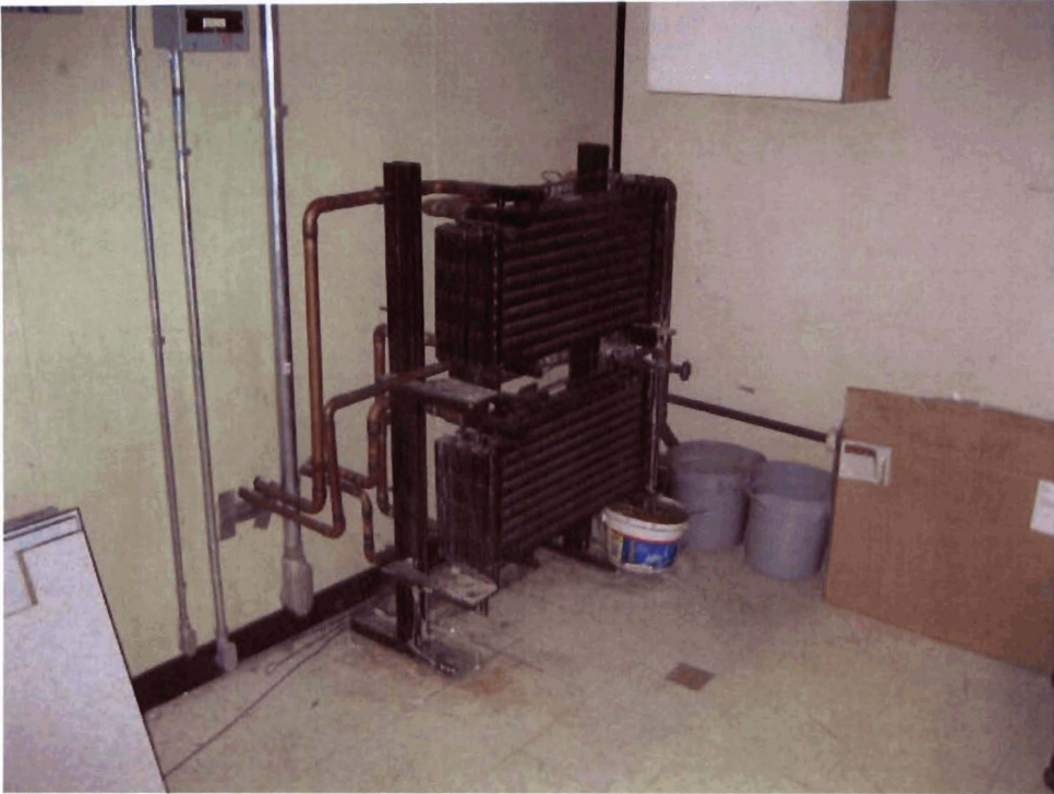
Photo 3: Existing IT Server Room AC Unit Heat Exchanger
